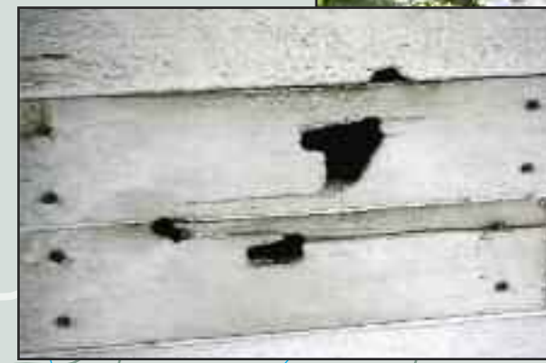
The Cannon Ball House in Blountville still shows shell damage to the exterior clapboard in the rear of the house.
